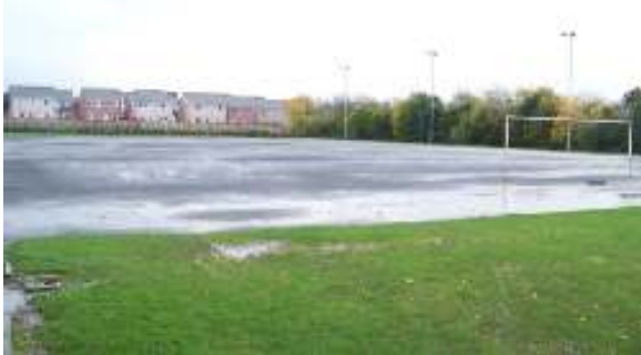
Flooding on Ash Park
